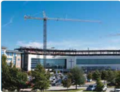
Tower cranes mean progress for Methodist Richardson's vertical expansion, which will add fifth and sixth floors to the hospital.
